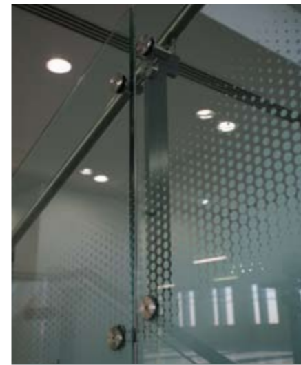
The glass extends above the handrail and is offset in front of the stair string.
