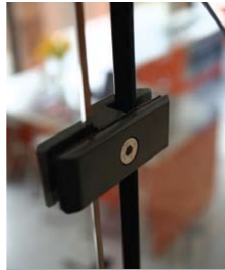
The glass balustrade is set within a pair of strings and, with no handrail, small joiners have a minimal effect on the overall appearance.
