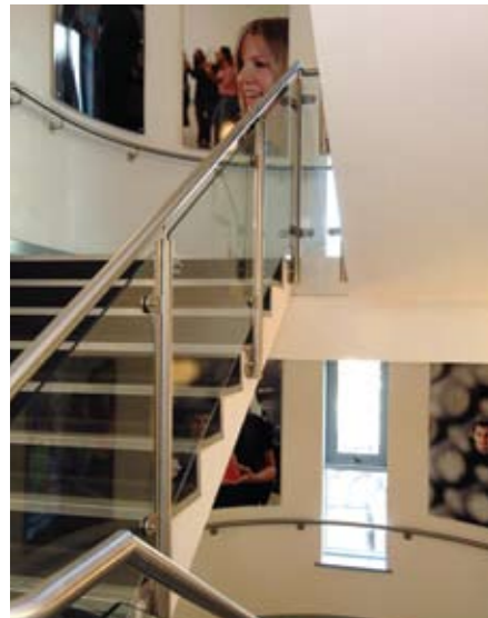
Internal stainless steel balustrade with glass infill panels, give a long term solution with minimal maintenance.
