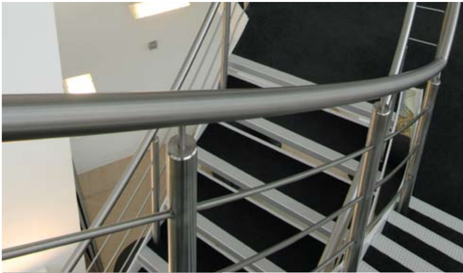
The satin finished stainless balustrade was installed as a final item and any isolated joints blended by our skilled installers.
