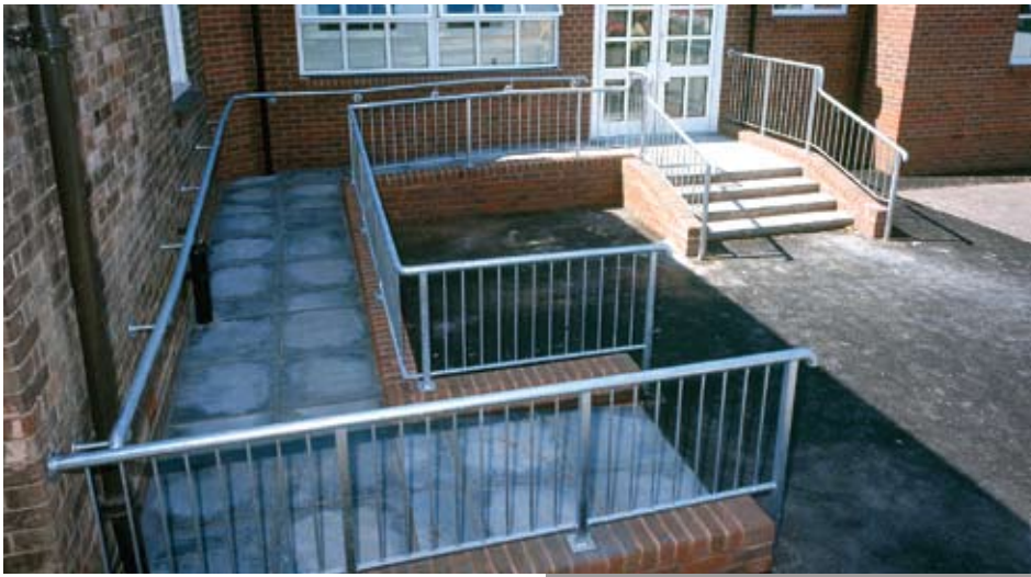
Mild Steel vertical bar infill ramp guard rails.
