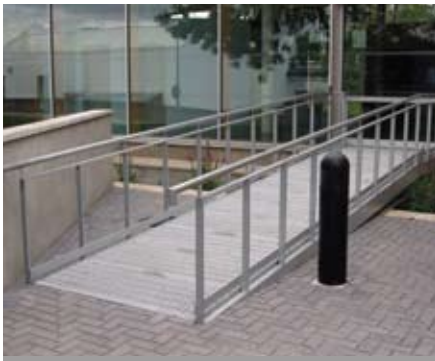
Disabled ramp access with punched non slip decking.
