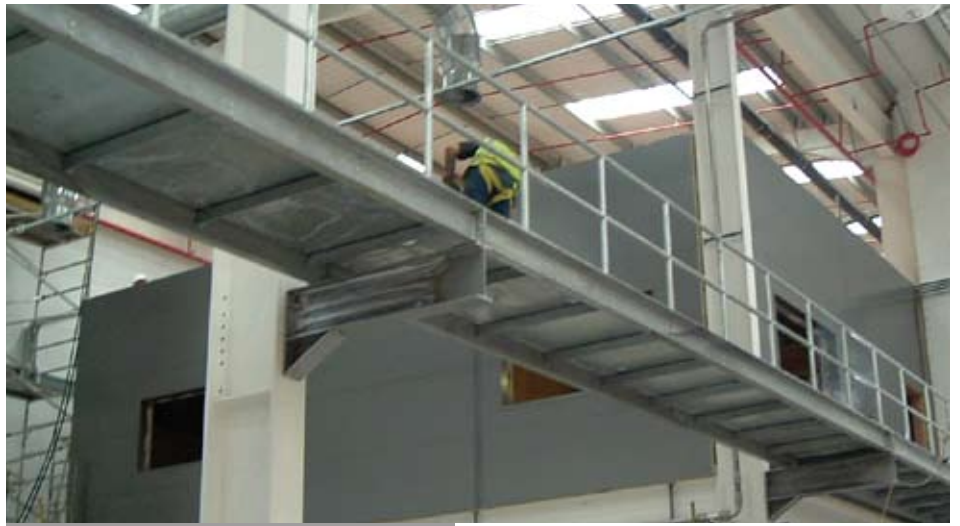
Industrial walkway with tubular guard rails.
